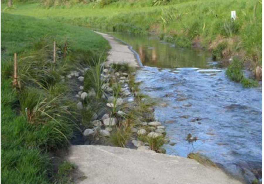
Fig. 3 Planted area and showing riffle created after placing rocks in concrete channel, Naenae
